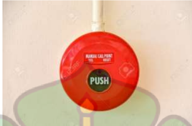
Gambar 5. 37 Fire Alarm Button
