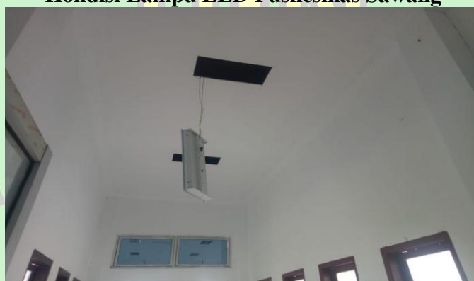
Gambar 4.6 Kondisi Lampu LED Puskesmas Sawang
