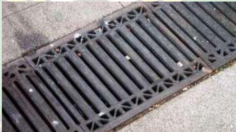
Gambar 4. 21 Grill Cover Drainase
