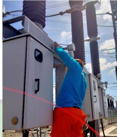
Pengecekan Bushing Transformator
