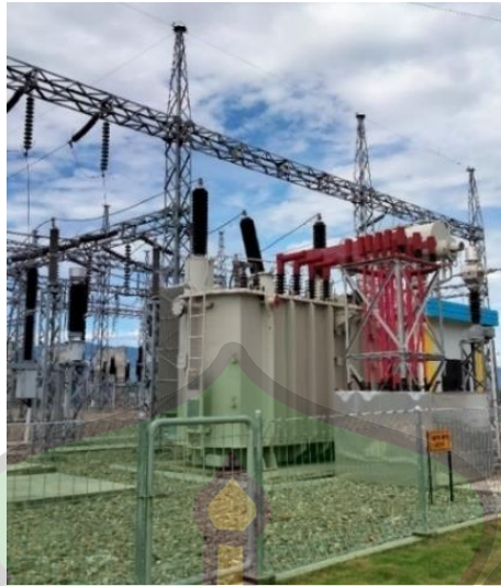
Gambar 2.3 Transformator Daya 60 MVA
