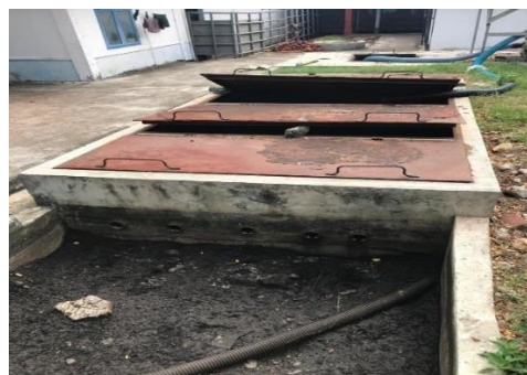
Gambar 3.5 Outlet IPAL RPH Gampong Pande
