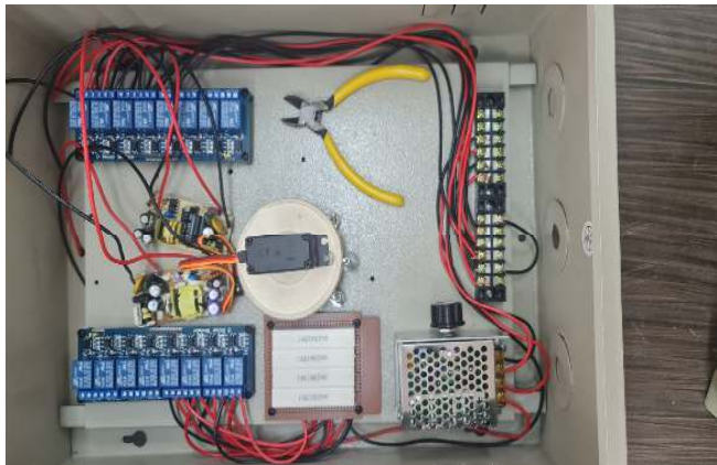
Figure 2. Components Inside the Panel Box for Digital Twin Technology
