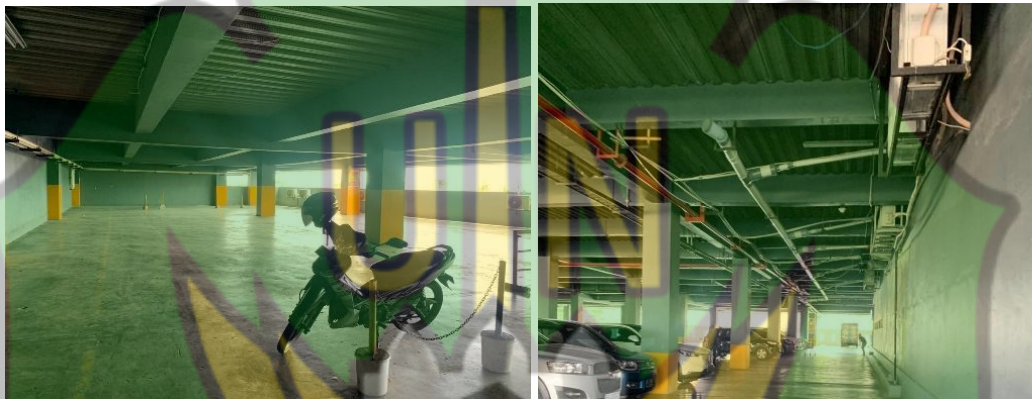
Gambar 4. 25 Plafon area basement existing tanpa sprinkler Sumber : Hasil Observasi, 2026
