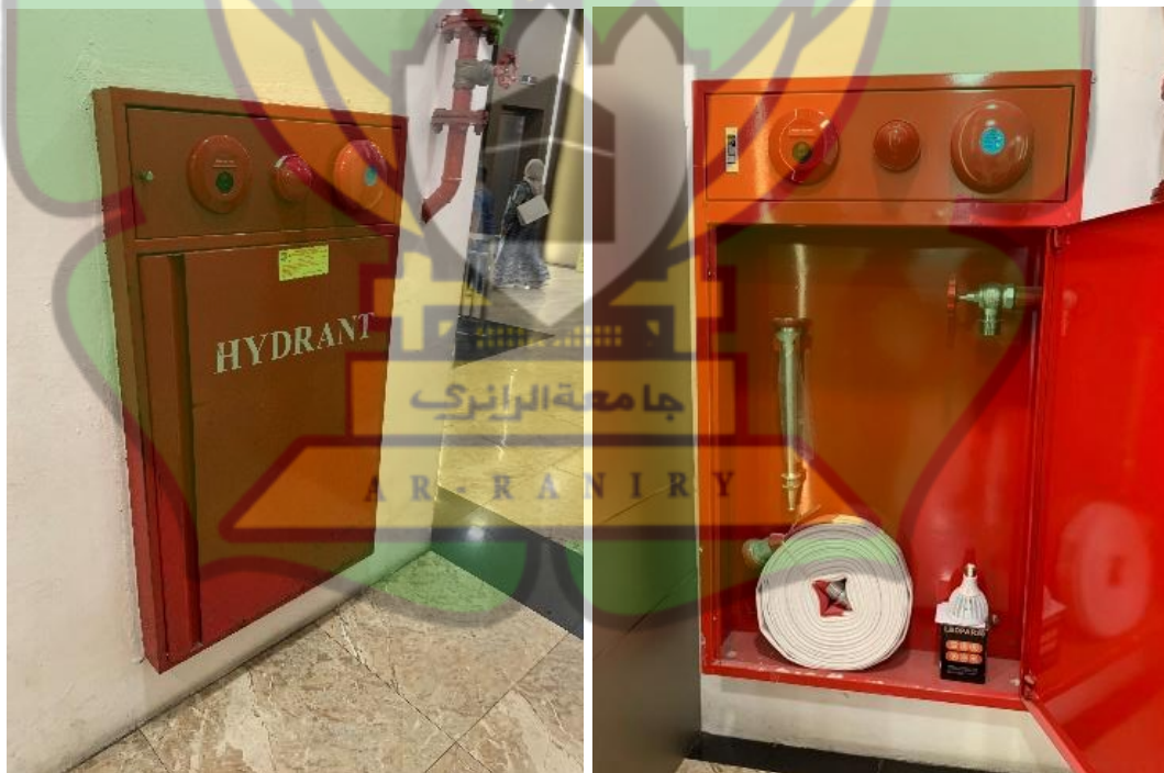
Gambar 4. 18 Hydrant existing Sumber : Hasil Observasi, 2026
