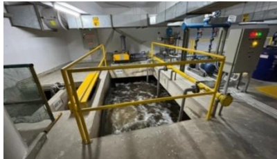
Gambar 4. 11 STP ( sewage treatment plant ) Sumber: Dokumentasi Pribadi
