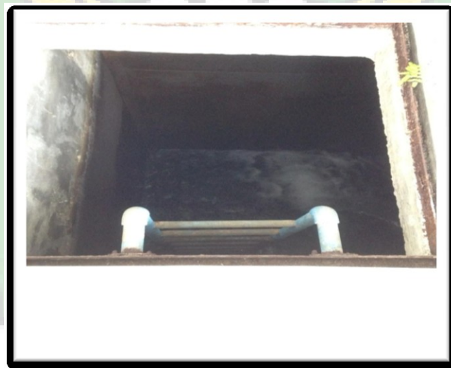
Gambar 4.10. Bak Reservoir Intake IPA Pria Laot
