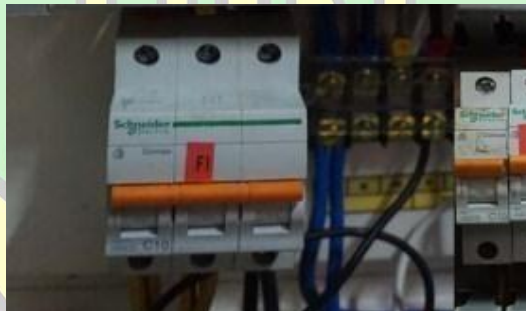
Gambar 2.1 Miniature Circuit Breaker (MCB)
