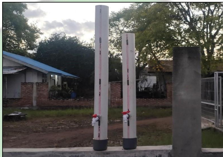
Gambar 4.1 Unit Filtrasi Rapid Sand Filter (RSF)
