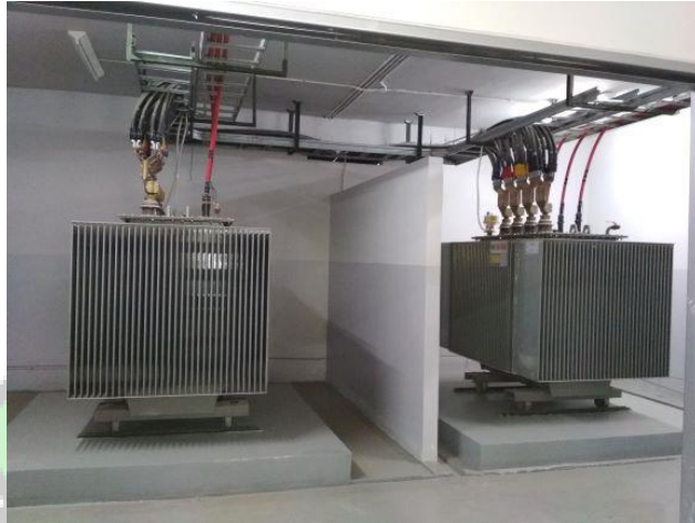
Gambar 4.28 Trafo Sumber: Wordpress.com
