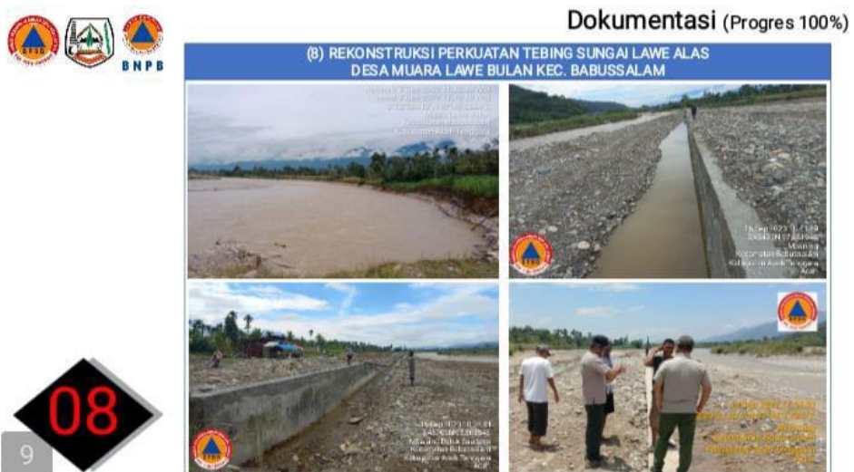
Gambar 5. Tembok Penahan Tebing Sungai
